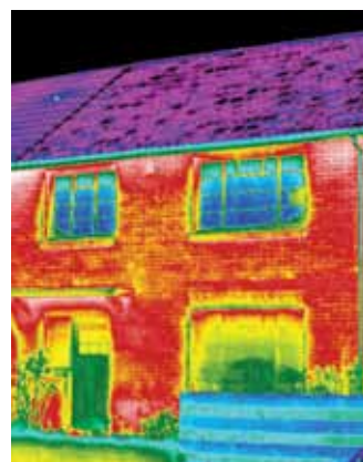
Substantial heat loss can occur through single skin walls. Photo courtesy of iRed Ltd
